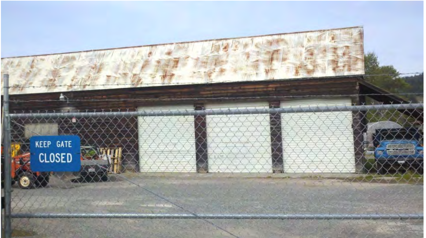
Photograph No. 23: Photo taken looking north at the City corporation yard shop, behind the chain link fence.
