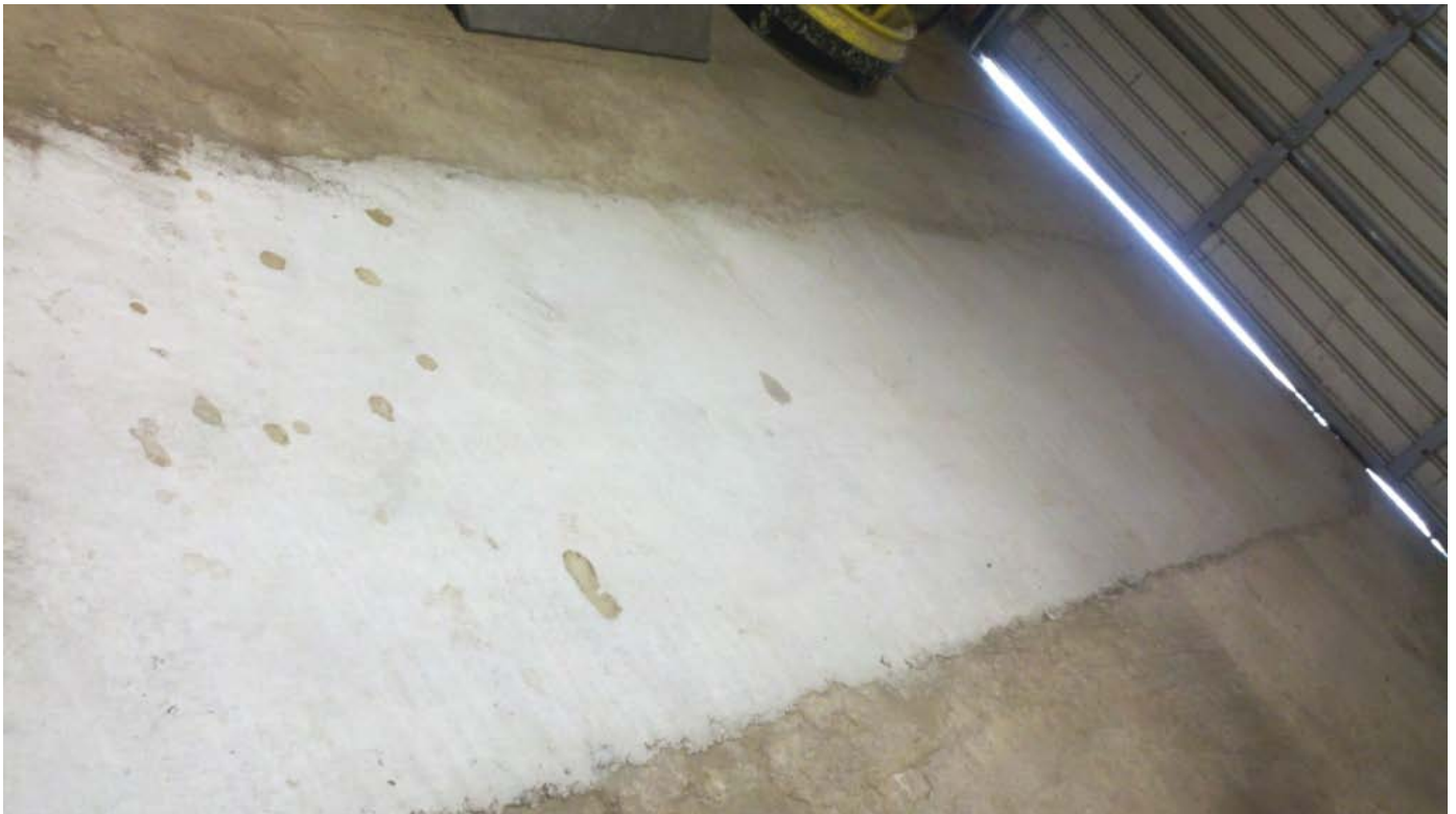
Photograph No. 24: Photo taken inside the first bay of the shop. There was once a mechanics pit, which is now filled with concrete.
