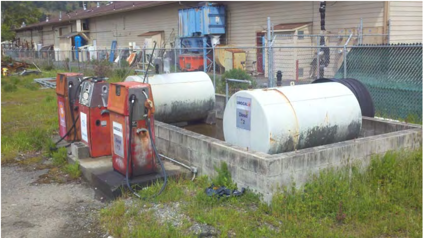
Photograph No. 29: Photo taken looking at the gasoline and diesel ASTs inside the concrete block secondary containment. There are three dispensers present, but only two are connected.
