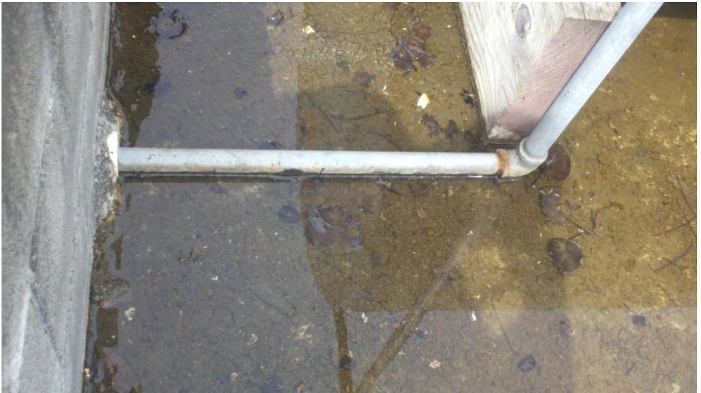
Photograph No. 30: Photo taken of the aboveground piping to the dispensers, within a second outer pipe, as it passes through the concrete to the dispenser.
