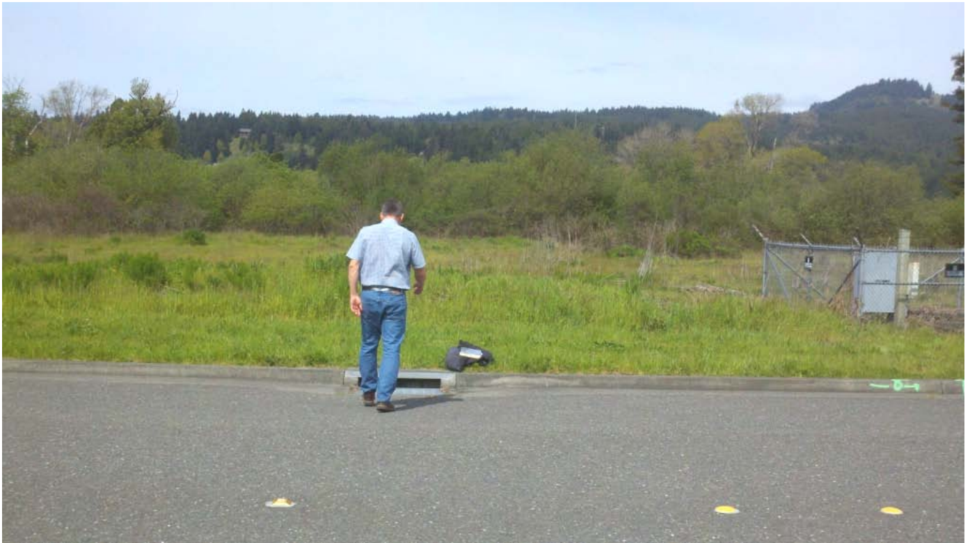
Photograph No. 9: Photo taken looking north at the storm drain drop inlet on Taylor Way. There is a storm drain that traverses between the two City parcels and discharges north into the creek.
