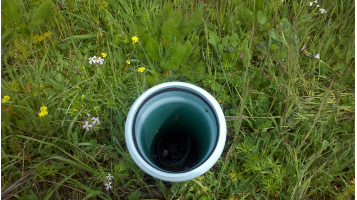
Photograph No. 13: Photo taken of a green pipe over a cleanout plug (APN 025-201-006).
