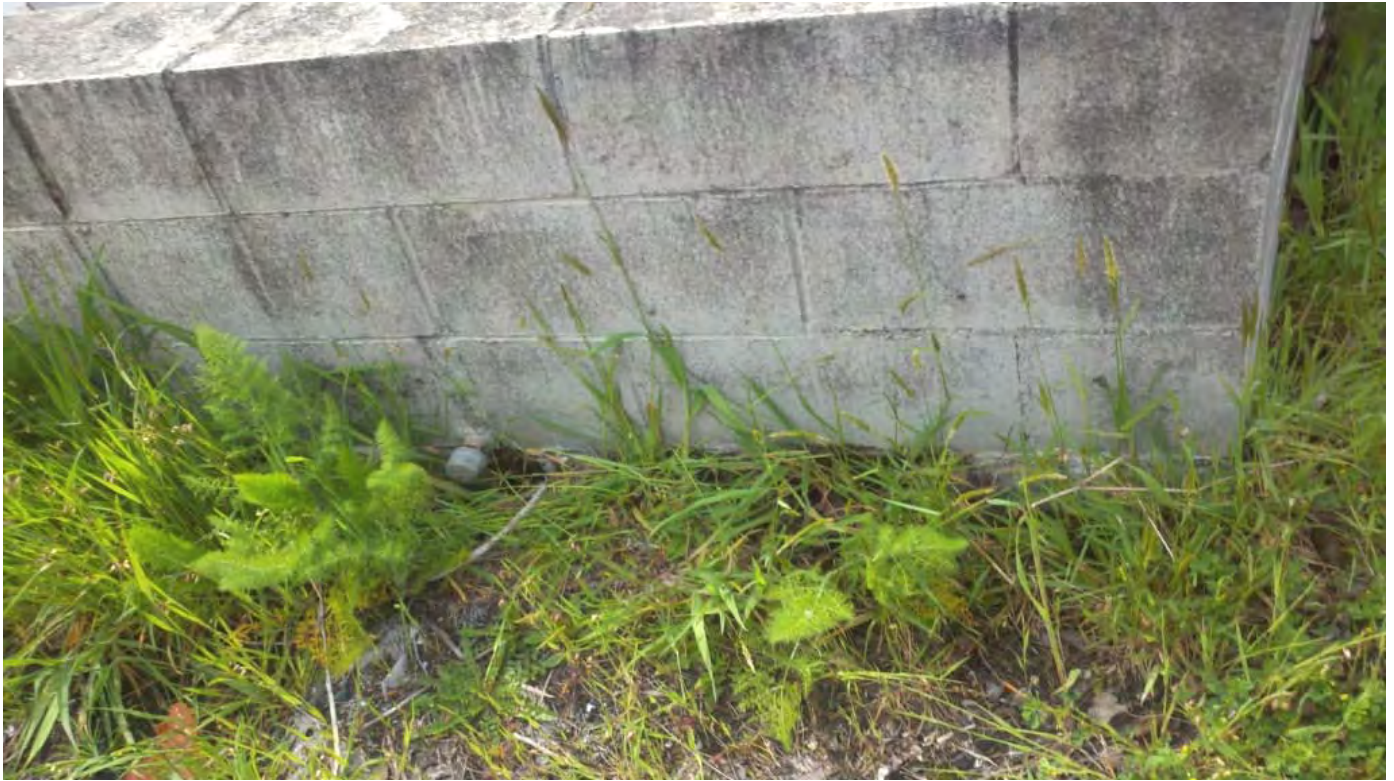
Photograph No. 31: Photo taken inside the City corporation yard. There are ASTs at the site; this photo shows the secondary containment drain valve that is capped.
