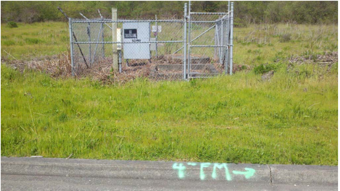
Photograph No. 7: Photo taken from Taylor Way looking north at the City pump station, which is between the two City parcels (APN 312-161-015 and -018). There is a 4-inch force main along Taylor Way, as well as other underground utilities.
