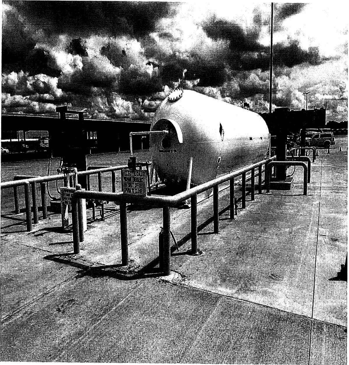
Image 30,000-gallon skid tank at school location
