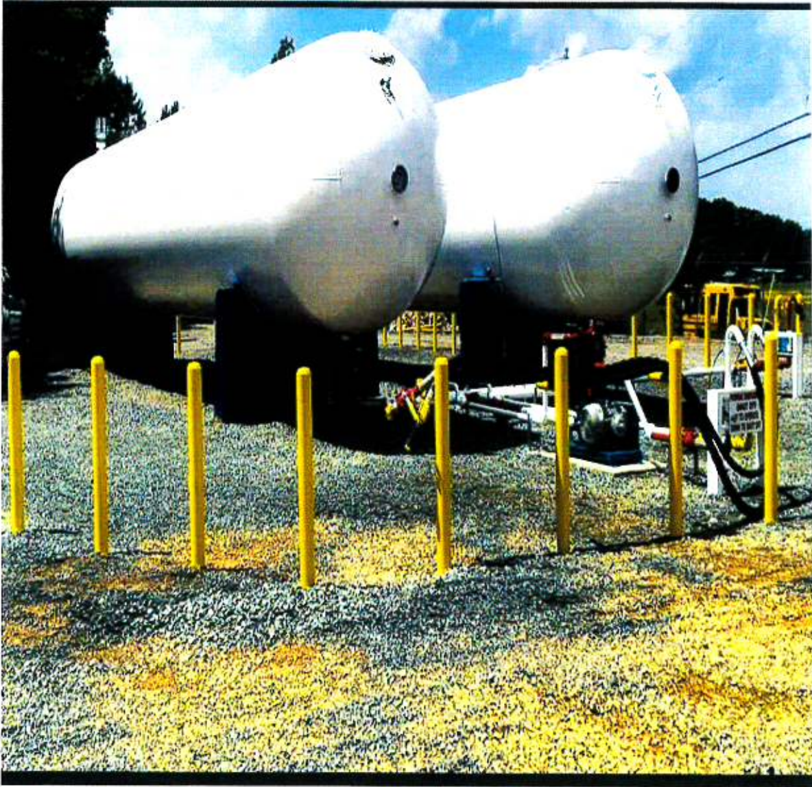
2-30,000-gallon tanks on piers with 4" bollards installed for vehicle protection.
