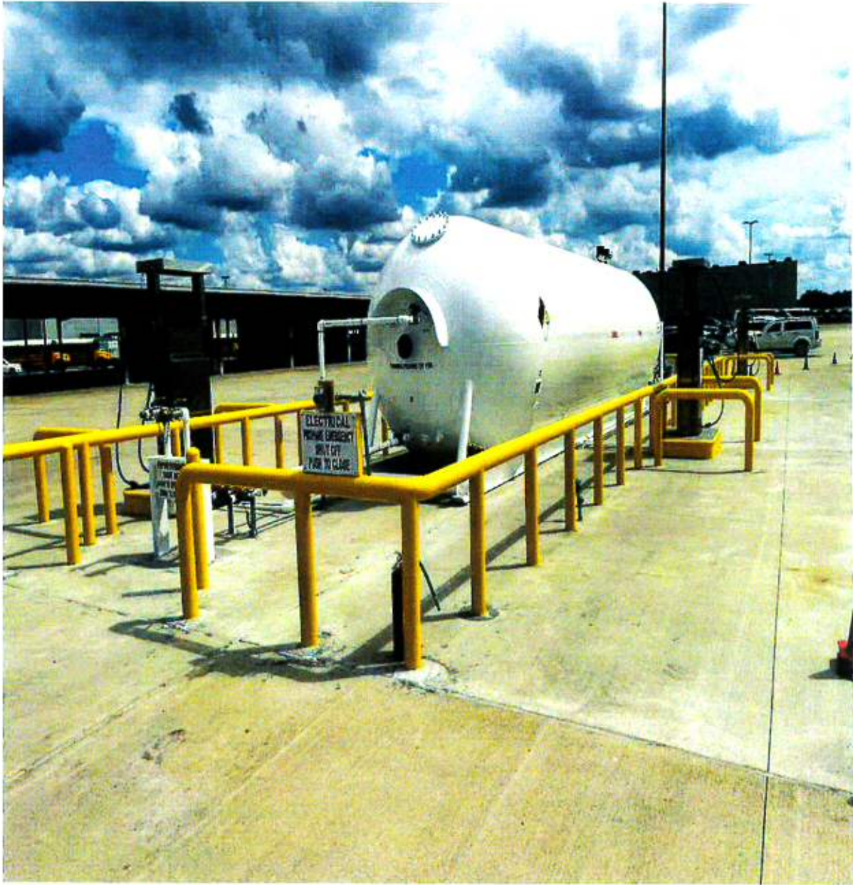
Image 30,000-gallon skid tank at school location
