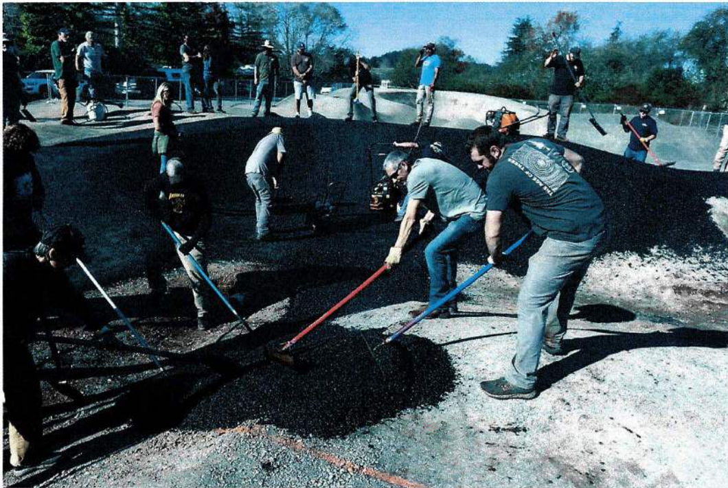
Volunteers spread asphalt Thursday in Blue Lake on a public skate/bmx park.
